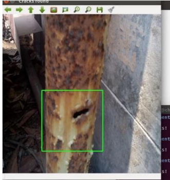
Figure 5.3. Example 2 for Crack Detection using Haar Cascade
